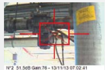
Picture of air leak localization
